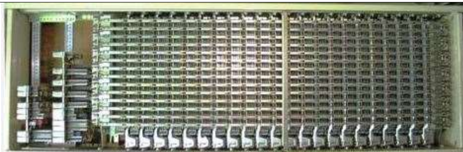
Figure 14—Pentaconta crossbar switch
