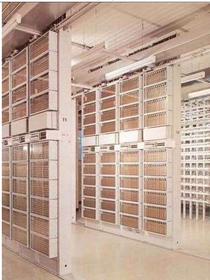
Figure 13—Ericsson ARF exchange at Viborg Denmark
